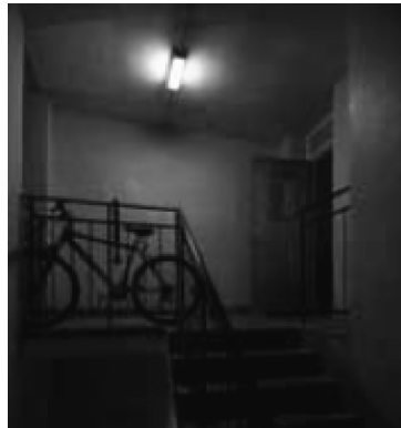
photo of stairwell with fluorescent fitting
